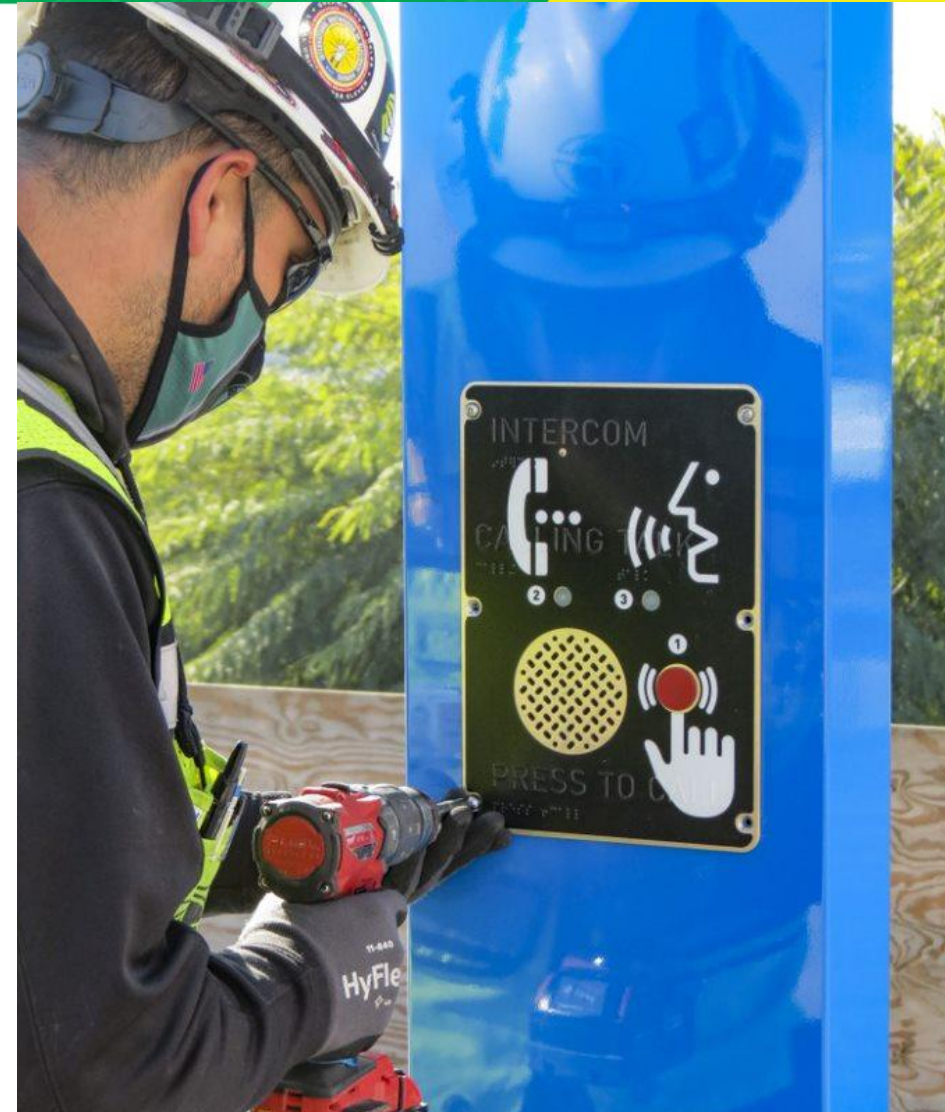
Blue emergency callbox on station platform installation
